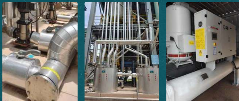
All Wilmar oleochemical plants in China have been upgraded to the Chiller Vacuum System, comprising of the Condenser System (top), Circulation Pump System (bottom left), Hot Well Unit (bottom center) and the Chiller Unit (bottom right).
